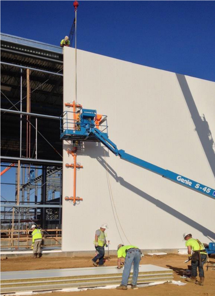
Figure 7: Installation of insulated metal panels (IMPs) with a non-combustible stone-wool core: factory-fabricated panels provide integrated air, vapor, water, and thermal barriers, enabling rapid on-site erection while enhancing passive fire resistance.
