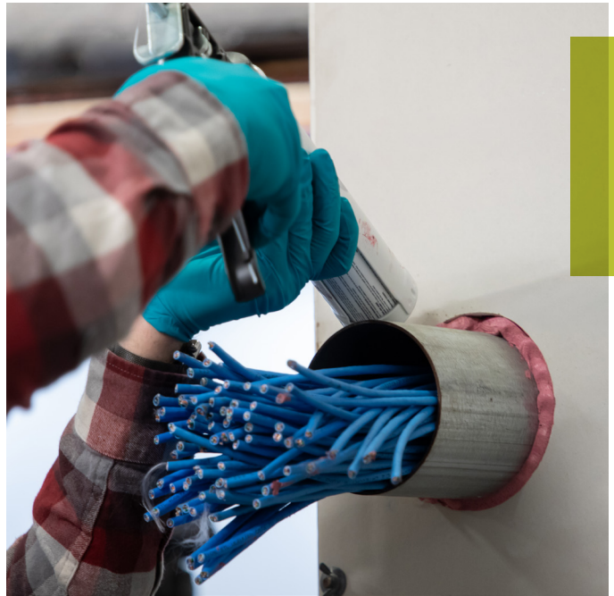
Figure 3: A mineral wool forming material is commonly installed within penetration openings and then sealed with a compatible fire-stop caulk.
