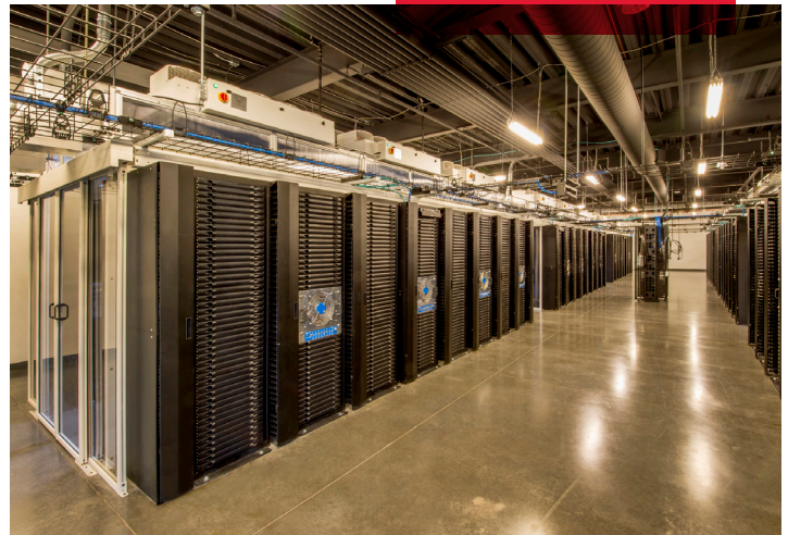
Figure 1: Interior of a modern data center with rows of high-density server racks.
