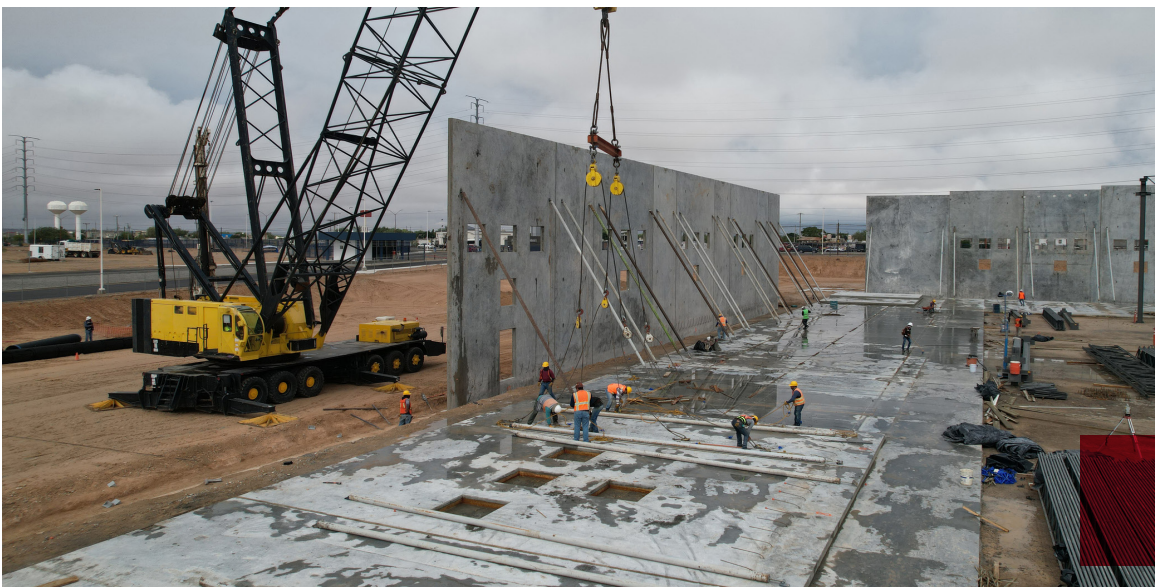
Figure 4: Tilt-up panel erection: site-cast concrete wall panels cast horizontally, lifted into position to form the building enclosure.
